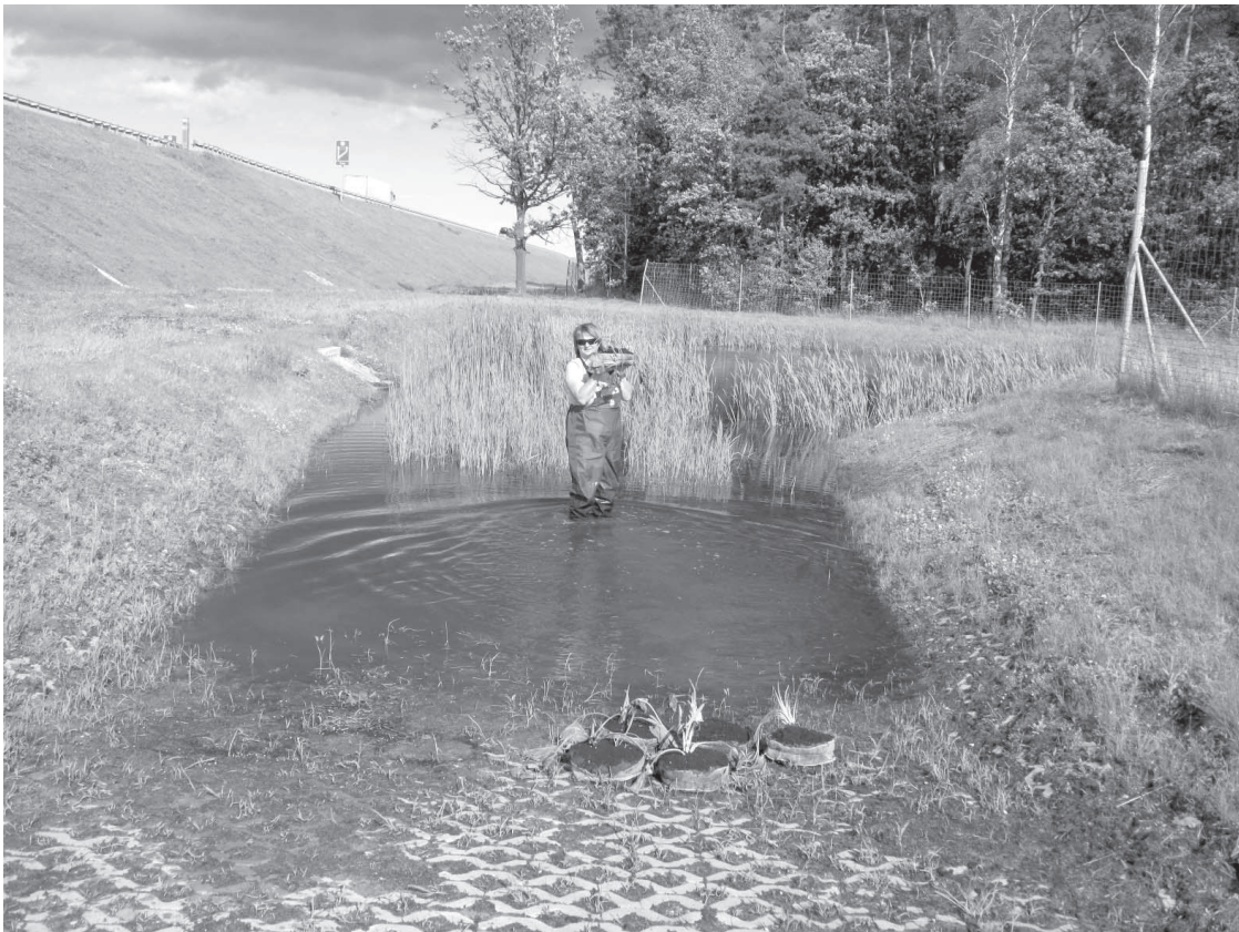
Fig. 2. Planting of the cuttings of Nuphar lutea in the settling basin in Dopiewo, at 147+100 km of the A2 motorway (photograph by J. Borysiak, May 2009)
